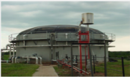
Figure 3b. The complete-mix digester at Oklahoma State University's Swine Research and Education Center.
