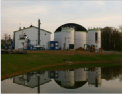
Figure 3a. The F550 system, quasar energy group's complete-mix digester at The Ohio State University's OARDC campus.
