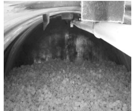
Figure 19. Examples of installations of premanufactured textile bioreactors. (Source: www.winnsystems.com )
