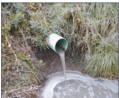
Figure 1. Liquid effluent contaminating surface water. (Photo courtesy of Rick Wilson, OEPA)
